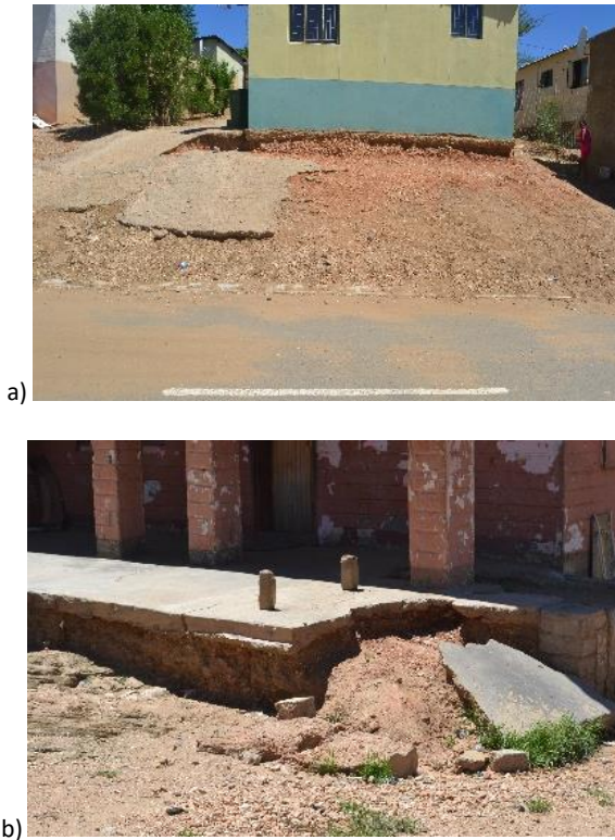
Figure 1: Examples of erosion damages to houses
